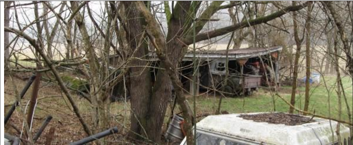
Photo 19: The Rocks, Jefferson County, WV View to southwest of fallen carport.
